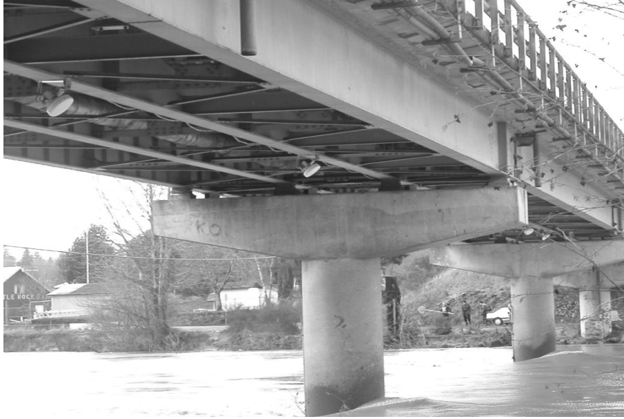
Figure 2: Four of the eight continuous wave microwave systems mounted on the Cowlitz River bridge at Castle Rock, WA.
