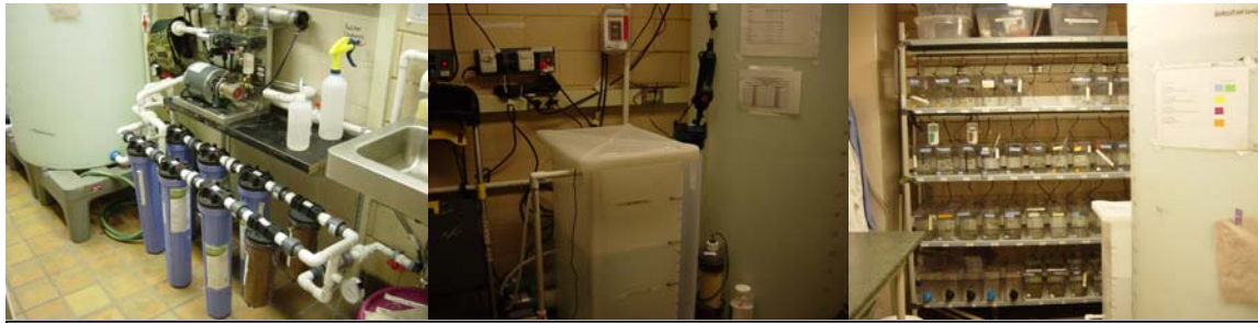
Figure 9.0 Left: primary filtration package Center: Salt sump Right: flow-through fish system
