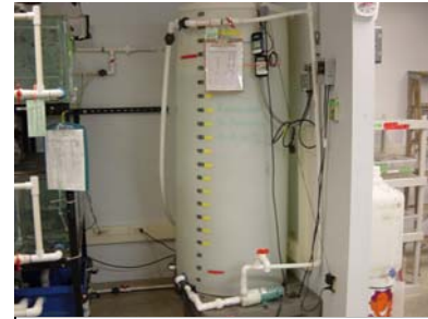
Figure 6.11 J083b laboratory system water tower.
