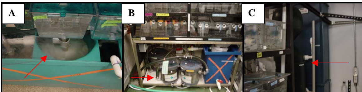
Figure 5.2 Red arrows indicate 3 different types of biofilters found in fish facility. A. Is a sand biofilter B. Is a polystrand pad biofilter C. Is an hour-glass bead filter.
